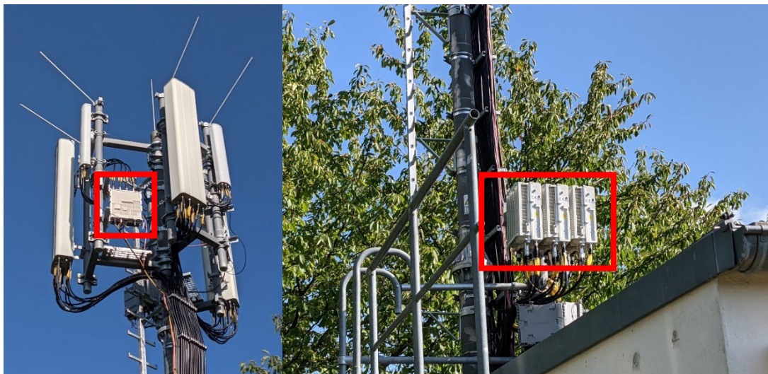
Figure 8: N78 5G Antenna External Macro Radio Unit & B7 LTE RRH in O-RAN Town (Fujitsu)
