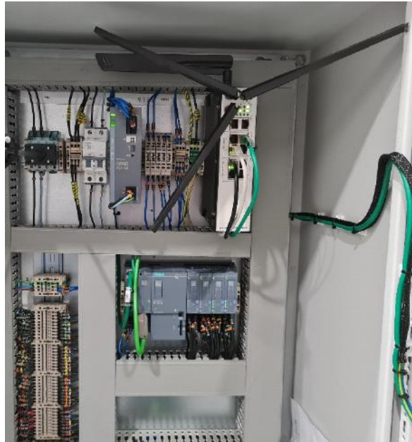
Figure 63: Furnace Monitoring Cabinet with NV1000 5G Router
