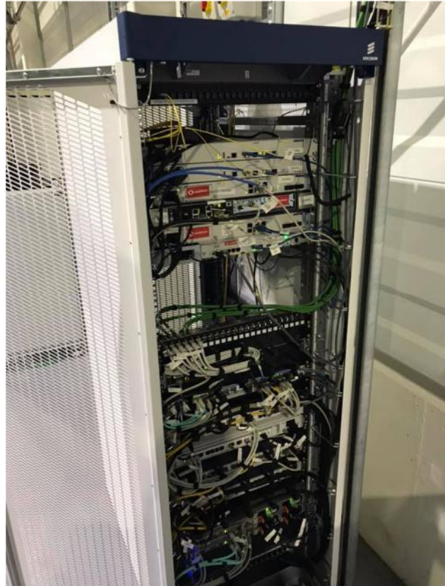
Figure 9: comms cabinet on Ford shopfloor.
