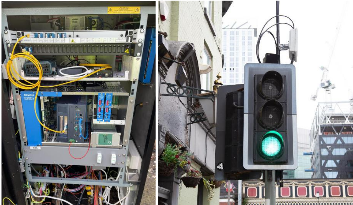
Figure 8: Installation of network hardware inside of Roadside cabinet & Benetel RAN650 small cell radio installed onto traffic signal pole using an extender pole
