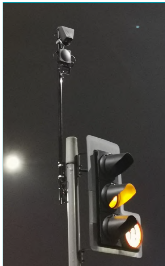
Figure 7: VivaCity Sensor installed using an extender pole onto a traffic signal pole
