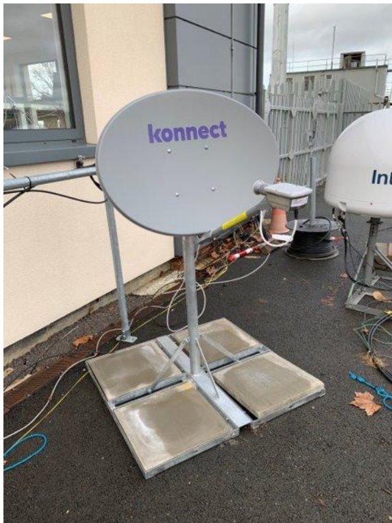
Figure 1 GEO terminal at Westcott
