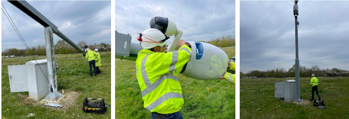
Figure 20 - CoMP-O-RAN Small Cell pole installation
