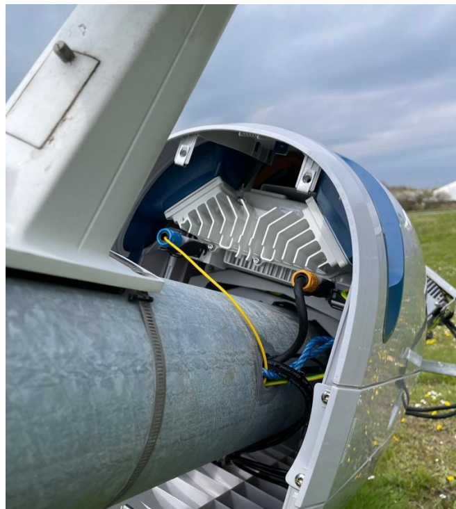
Figure 12 - Power and fibre cabling covered by the shroud
