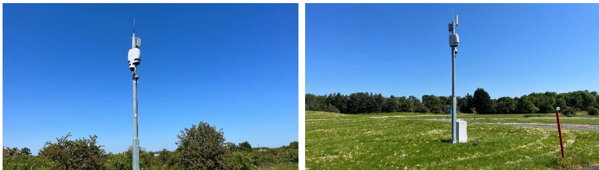
Figure 39 - City Course Masts with CoMP-O-RAN Small Cells
