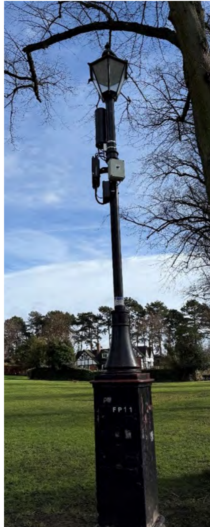
Figure 2. Small Cell attachment onto modified multi-functional column (Shropshire)
